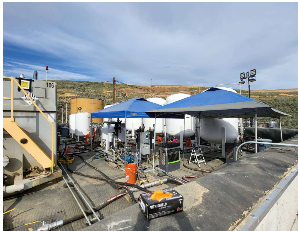
Photo 2: Overview of the liquid treatment area.
